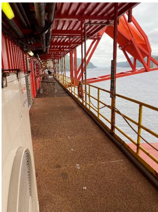
Figure 0-31: Escape ways missing yellow colour
