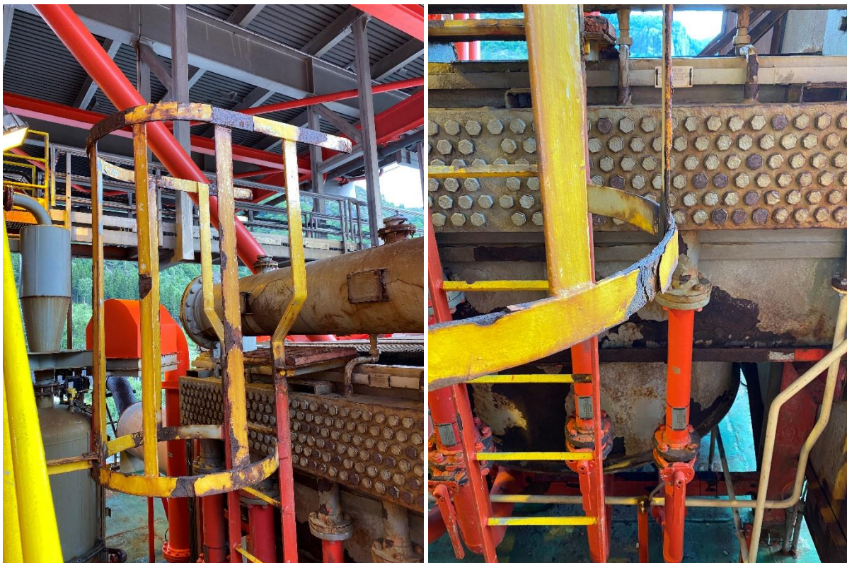
Figure 0-18: Safety cage on ladder could use some maintenance
